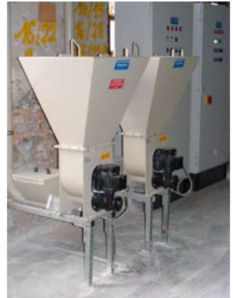
Dry feeders for the supply of calcium carbonate
