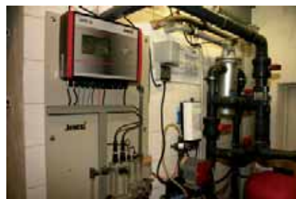
TOPAX® NT, MAGDOS LT and Technoline SC14 mounted on monitoring board PM01
